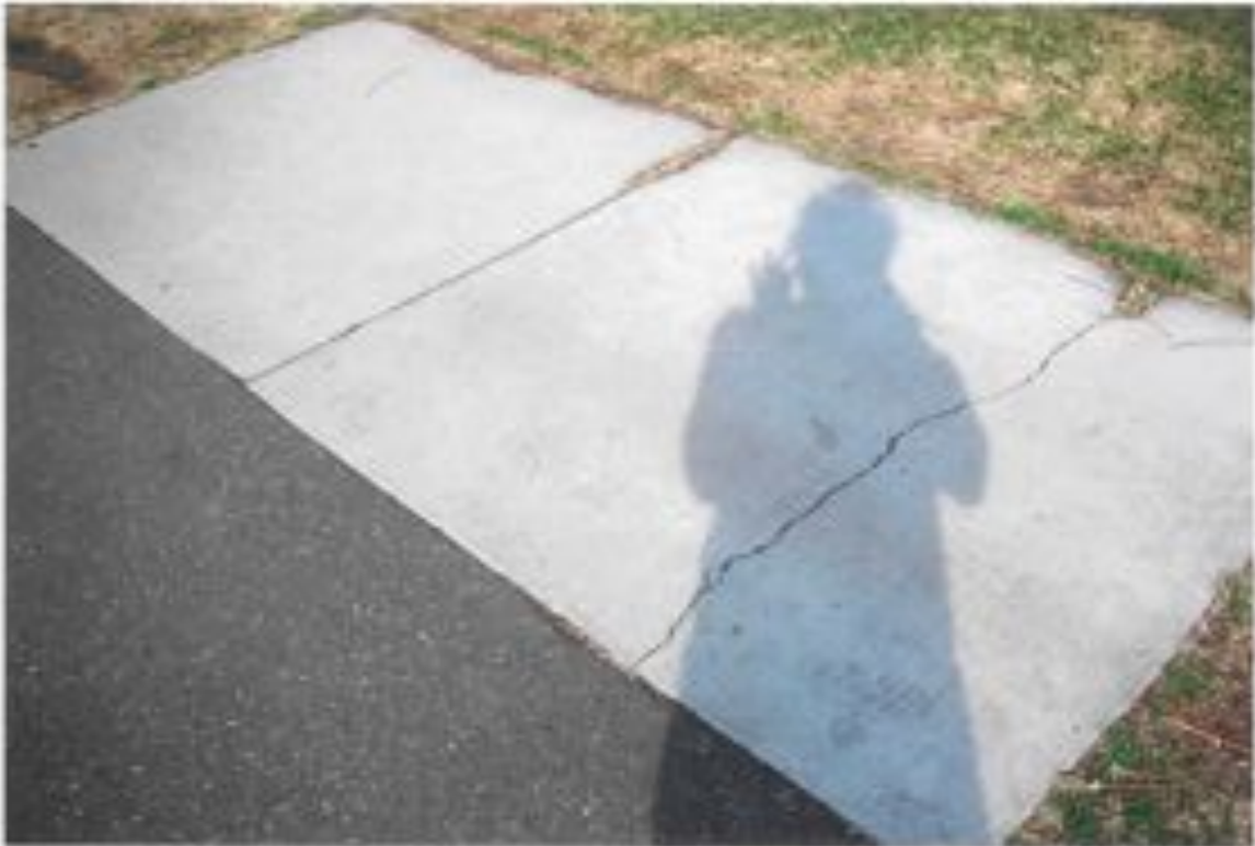
Benches Cracked concrete
