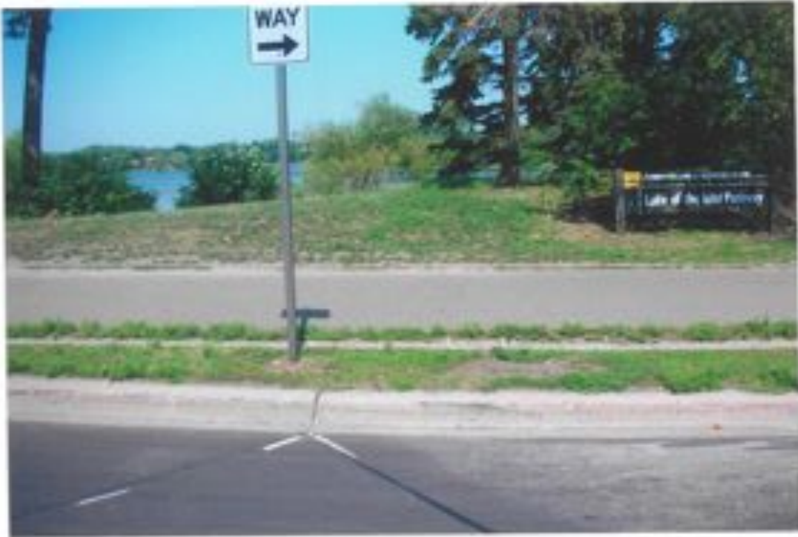
Gateway Intersection at E. Lake of the Isles Parkway & E. Calhoun Parkway Misplaced "LOI Parkway" and One Way signs
